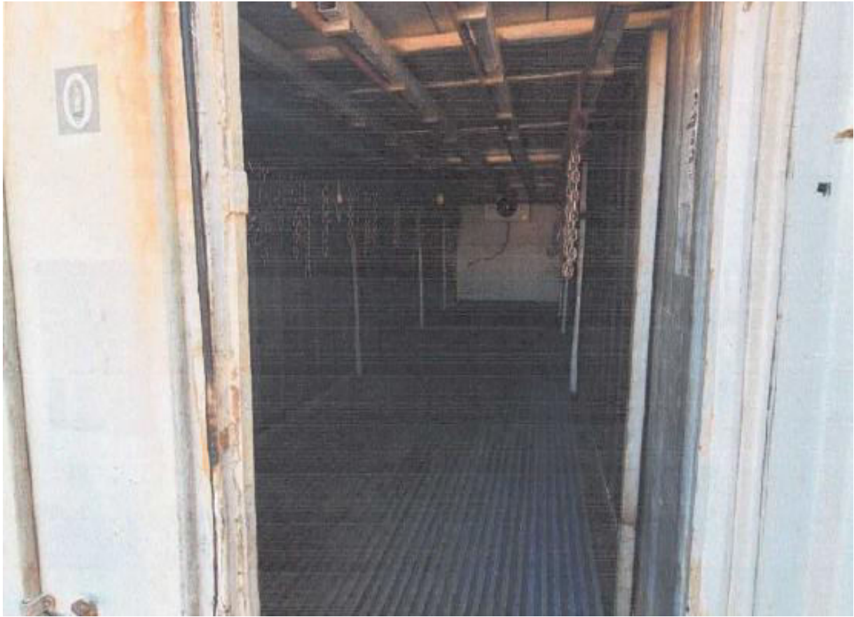
Figure 7: Internal View of Coolroom
