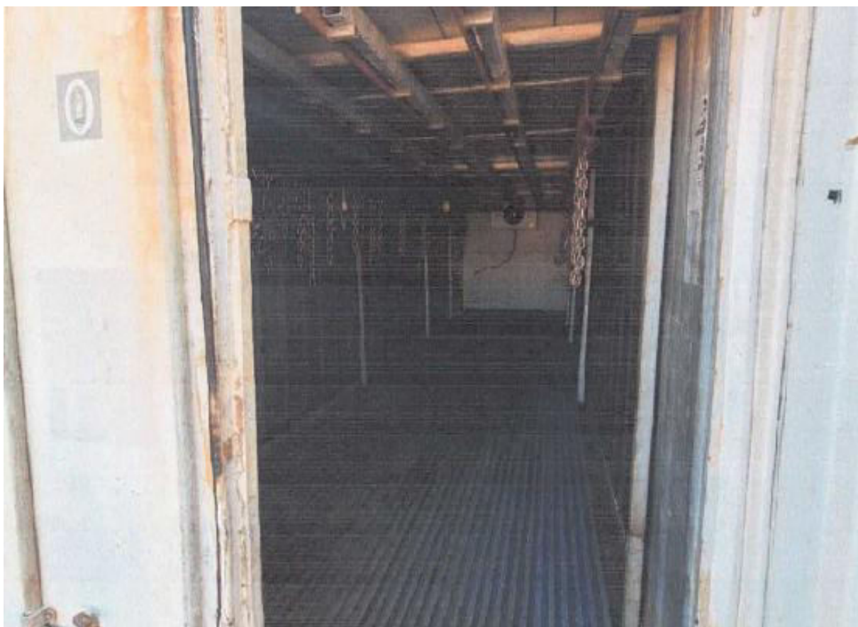
Figure 7: Internal View of Coolroom
