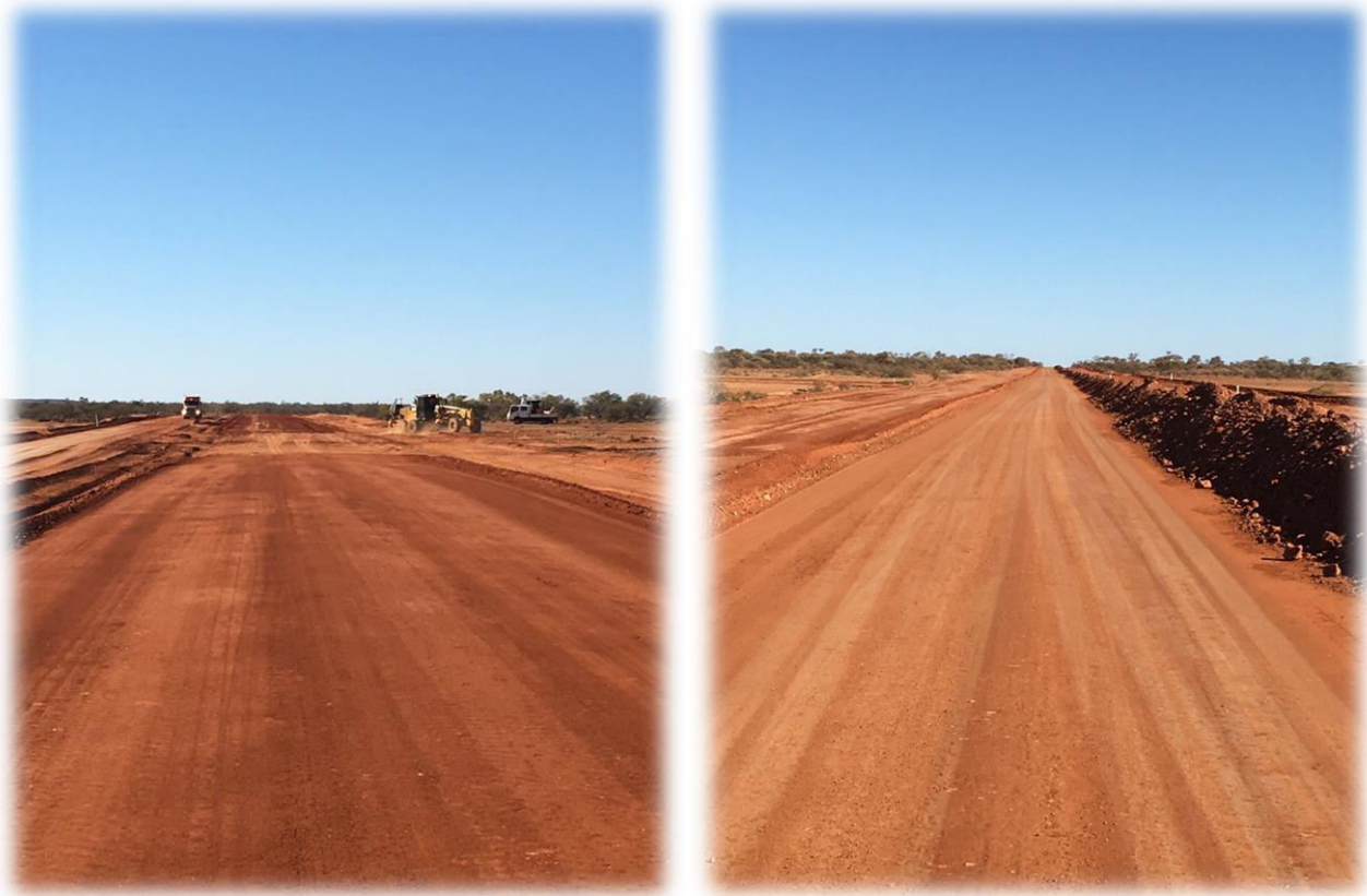
Figure 2: Flood ways boxed out and Sub grade ready for new base course
