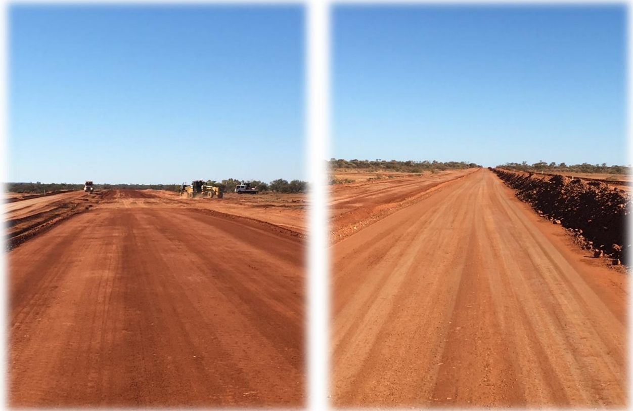
Figure 2: Flood ways boxed out and Sub grade ready for new base course
