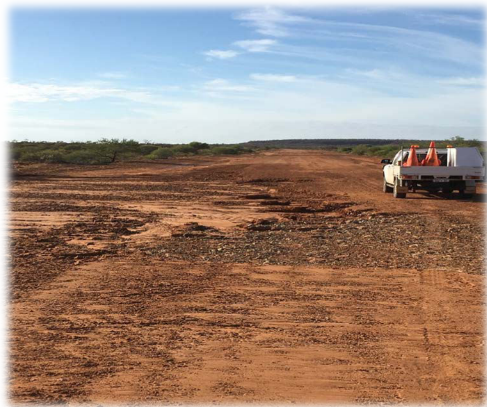
Figure 1: Minor damage near Pells Range
