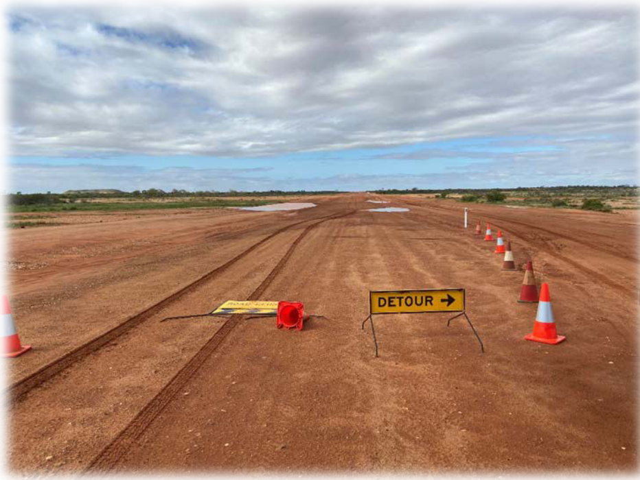
Figure 4 Road Closed sign run over and detour ignored on works prepared for bitumen
