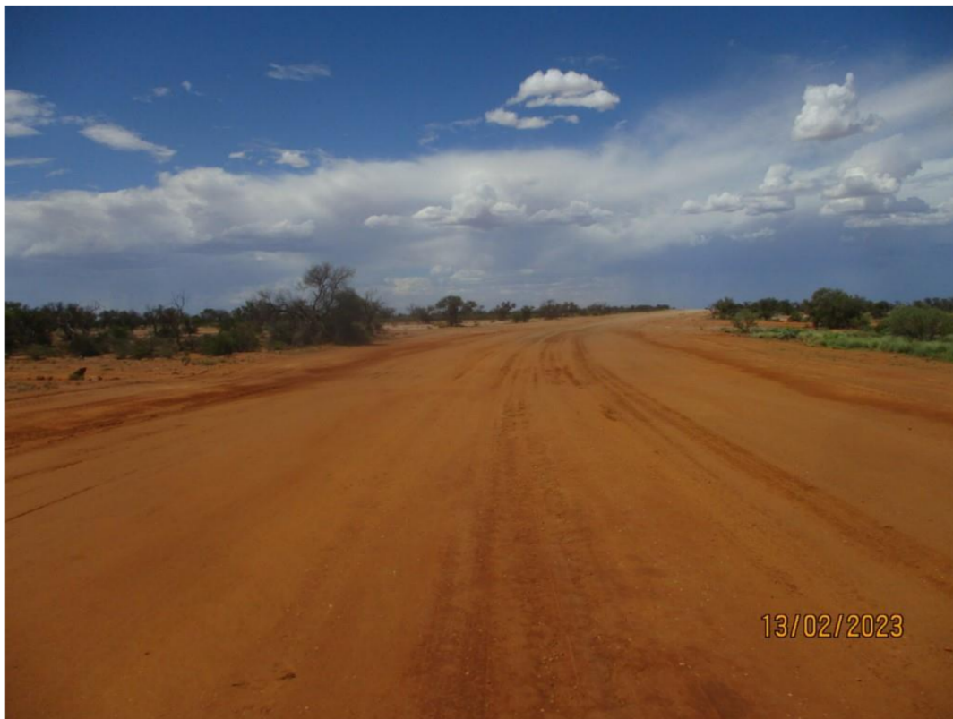
Figure 2: Cobra Dairy Creek Rd SLK 107 After
