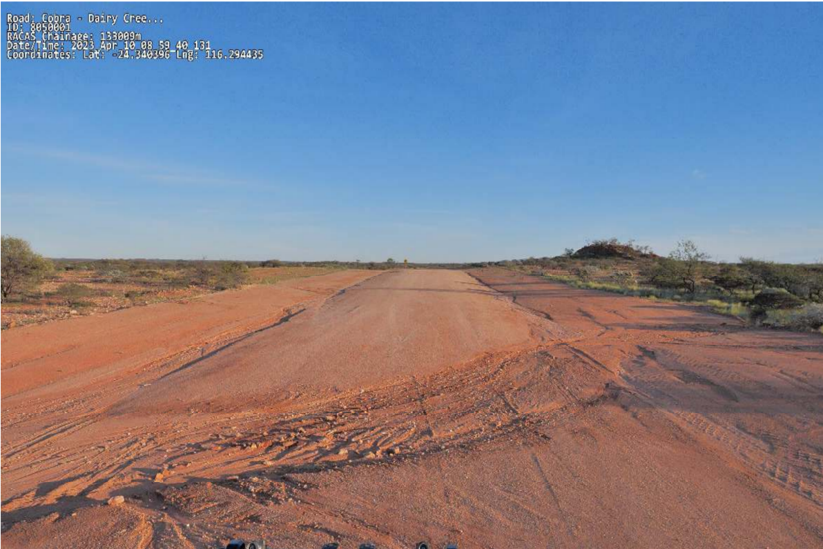
Cobra Dairy Creek Rd Slk 133.009-133.021 - Defect
