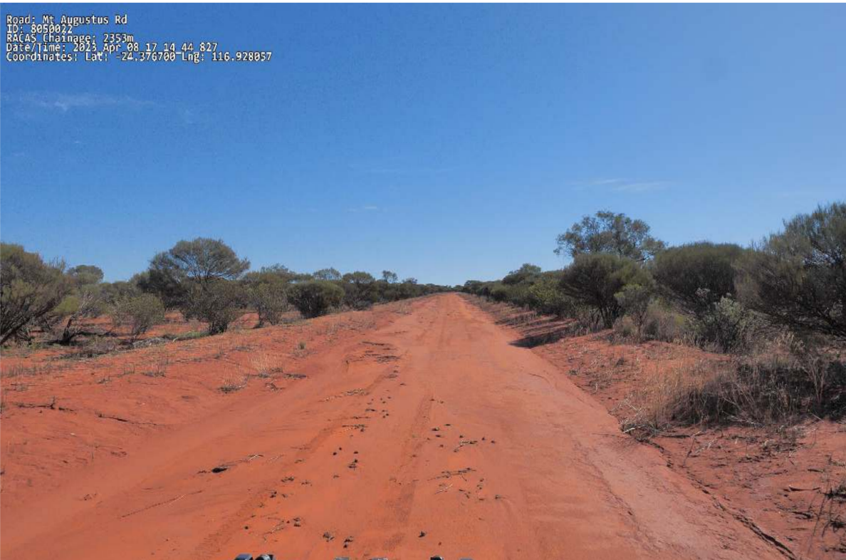
Mt Augustus Rd Slk 2.353-2.393 - Defect
