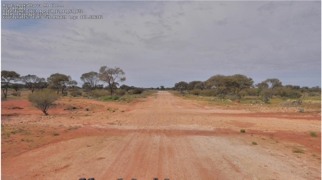
Meekatharra Mt Clere Rd SIK 0.331-0.354 – Defect
