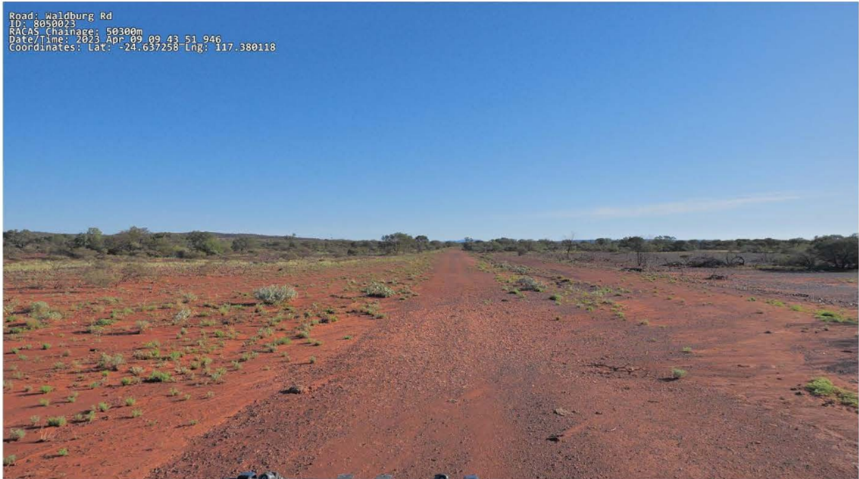
Waldburg Rd Slk 50.300-50.322 - Defect
